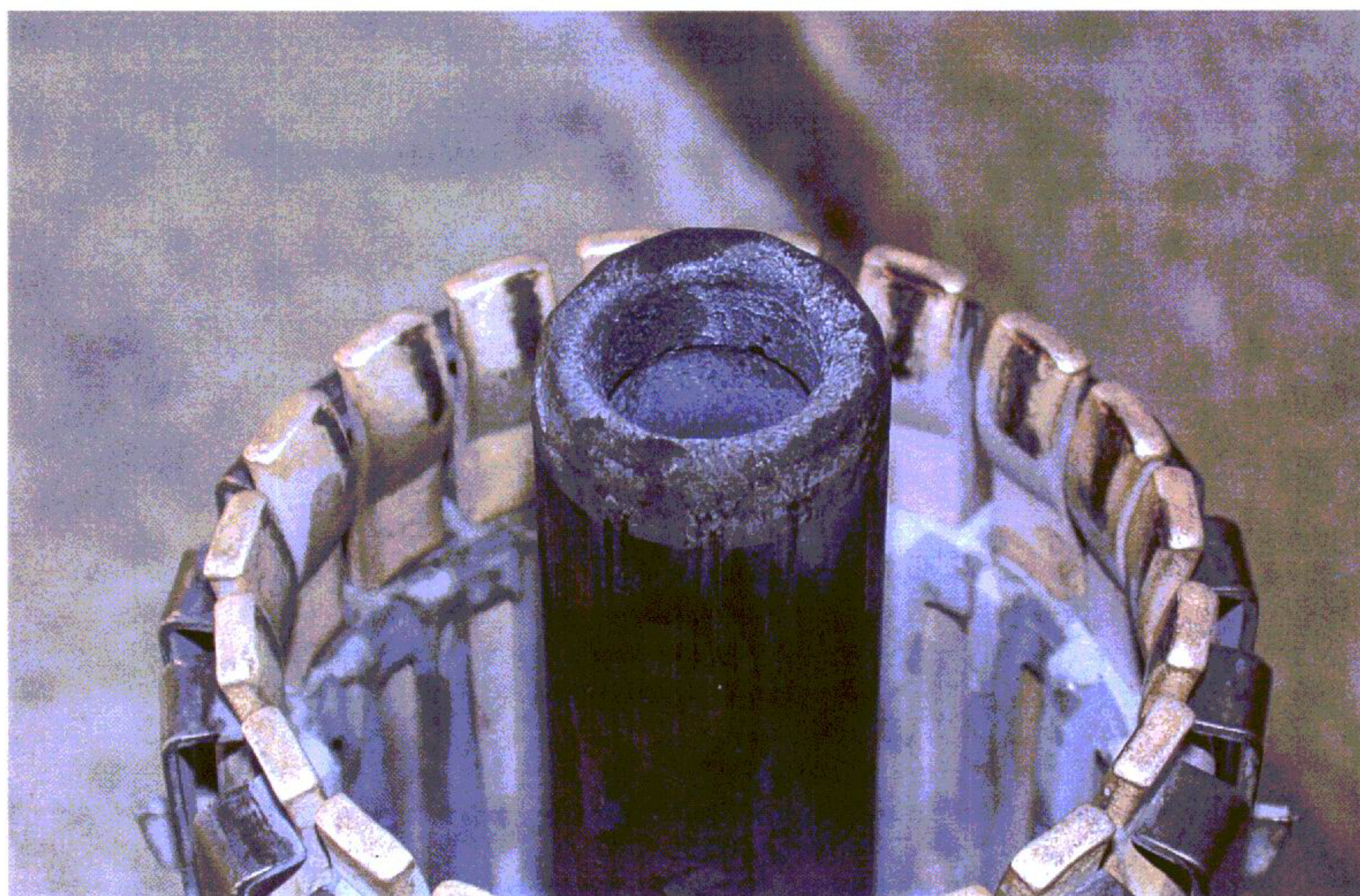
Photo no. 7 Phase S
